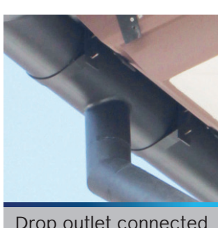
Drop outlet connected with downspout
